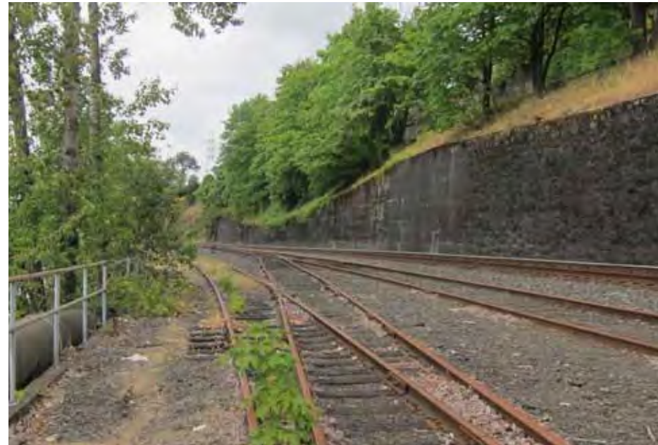
Rail spur south of site offers potential connection to Canemah and Metro Natural Area
