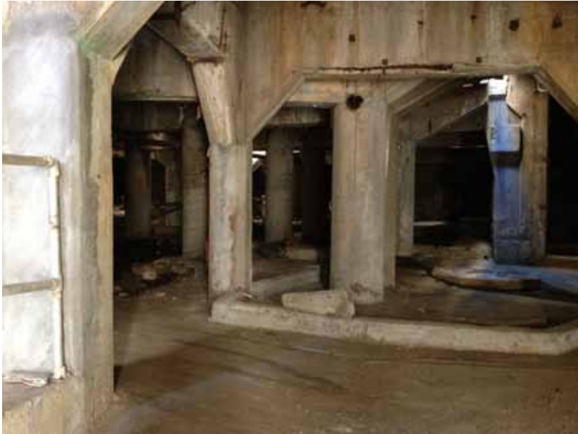
Many of the concrete mill structures have massive concrete foundation systems with interesting spatial qualities.
