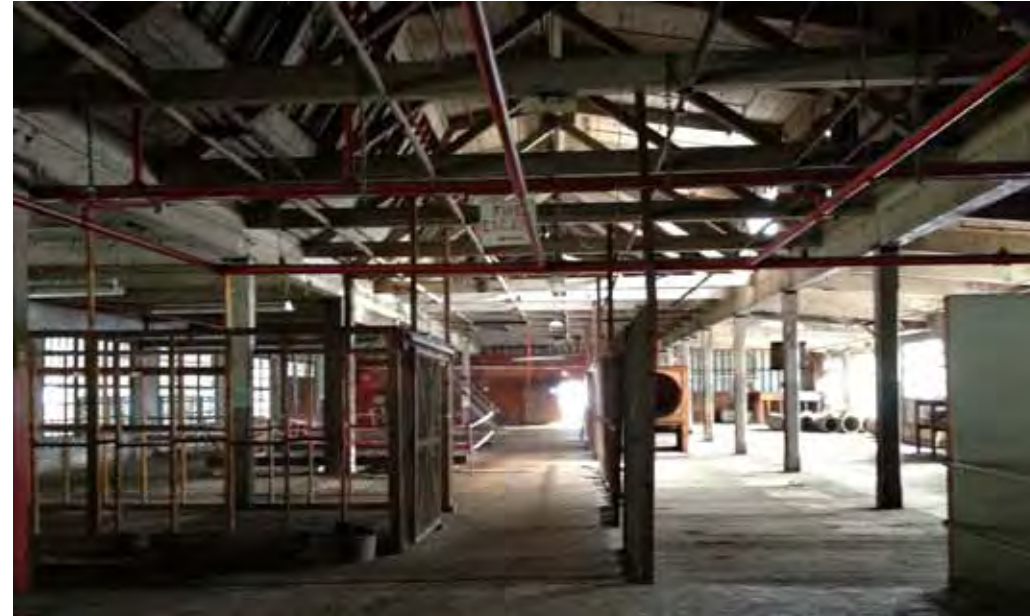
In addition to the massive concrete column and beam mill structures, wood framed buildings exist on site with exposed wood columns, beams, and roof trusses.
