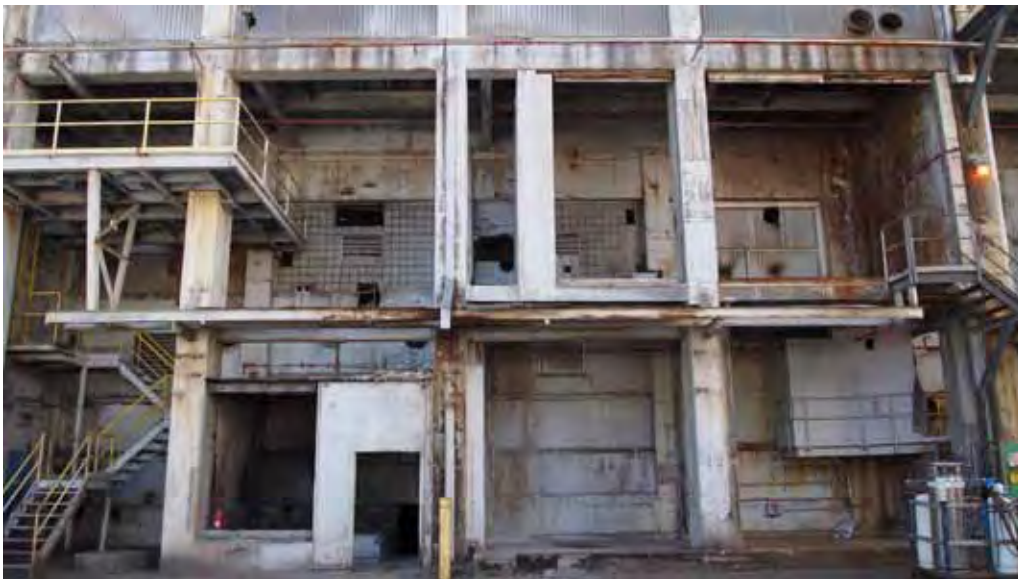
Even after the salvaging of materials, many of the existing mill structures retain an authentic industrial character.
